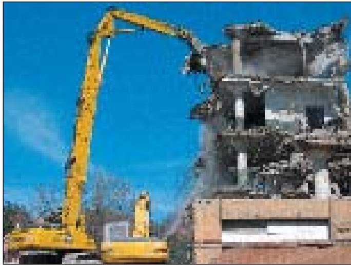
The building's proximity to the street meant J&B Construction and Services Inc. had to explore alternative methods of demolition.
