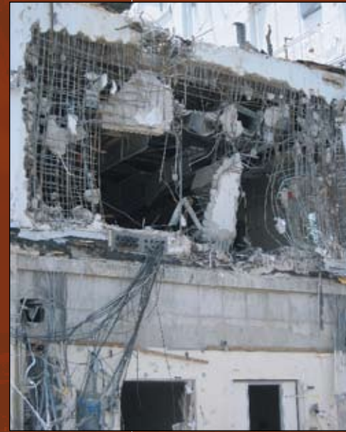
The high concentration of rebar in SAEF II was a challenge for the demolition team.
